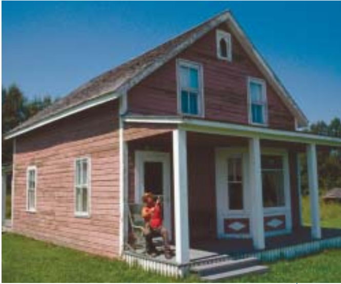
Sanding wood on front porch of house in Aroostook County, one of the 10 counties currently served by MCF's County Program.
